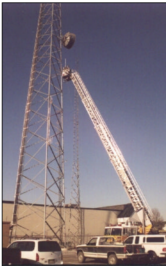
View of the antenna installation at the Augusta EOC Center in Verona.
