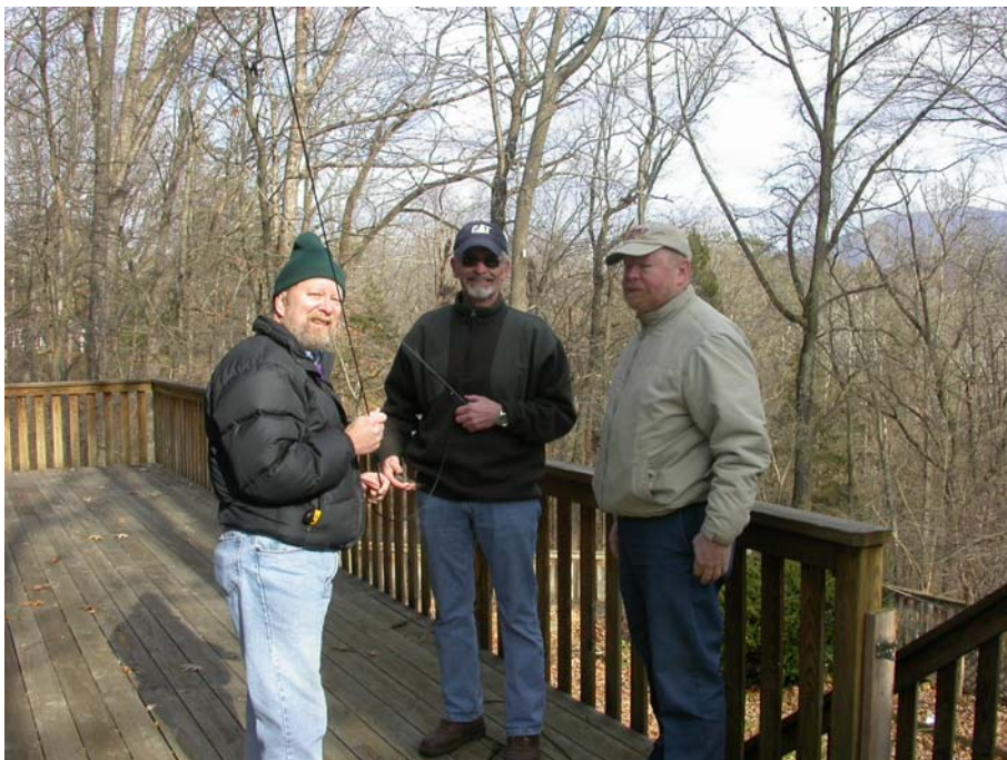
(Left to right) Dave/K4DPF, Mark/N4YSA & James/W4SIU - installing HF loop antenna at K4DPF's QTH on a cold, windy, blustery day.
